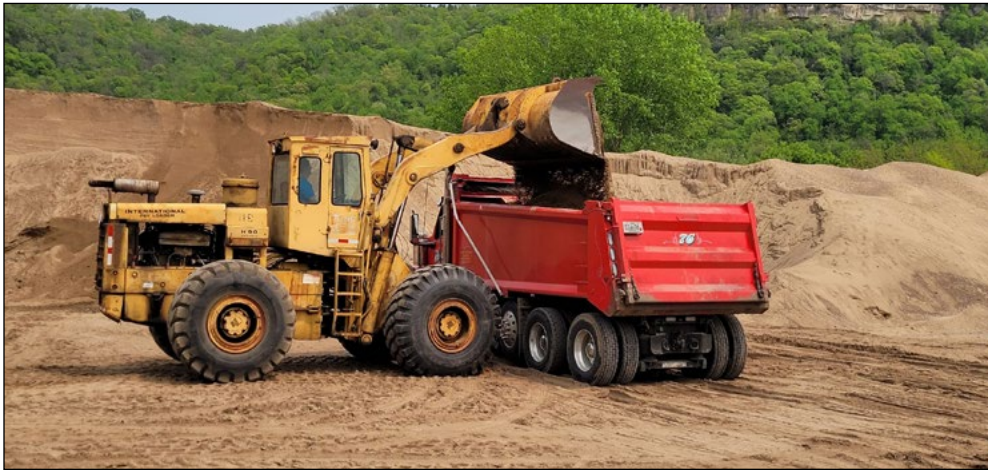
An excavator puts river sand into a truck, which will be used to fill sandbags, near Alma, Wisconsin, May 16. The river sand is available at the Alma Marina beneficial use site for the public. USACE St. Paul District photo by Elizabeth Stoeckmann
