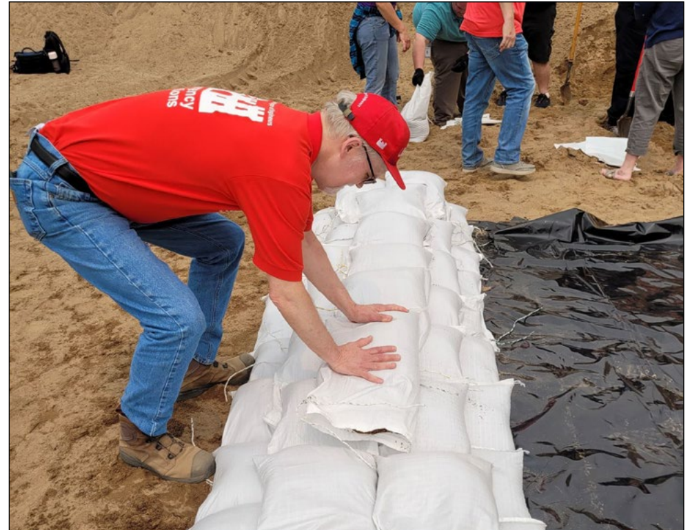
Scott Baker, Winona resident engineer, places sandbags at a sandbag training near Alma, Wisconsin, May 16. USACE St. Paul District photo by Elizabeth Stoeckmann
