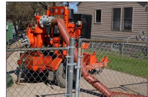
A pump and a hose in Campbell, Wisconsin, April 26. USACE St. Paul District photo by Elizabeth Stoeckmann
